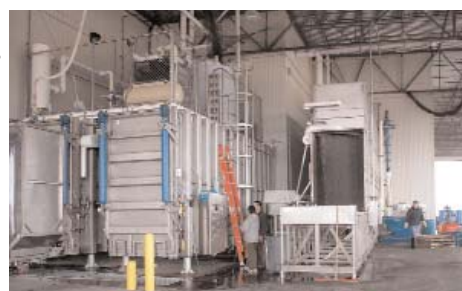
The new Hydro-Vac Machine, left, is being installed and checked by engineers
